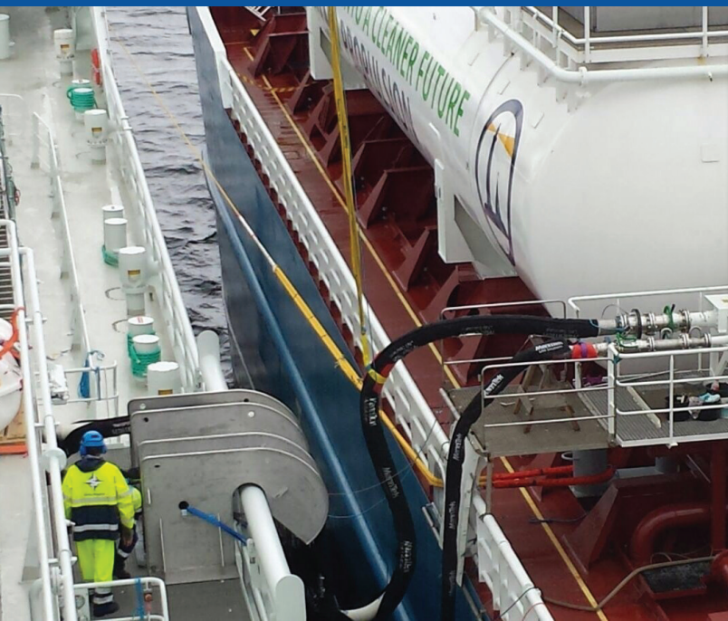
Coralius performs ship to ship LNG bunker operation.
