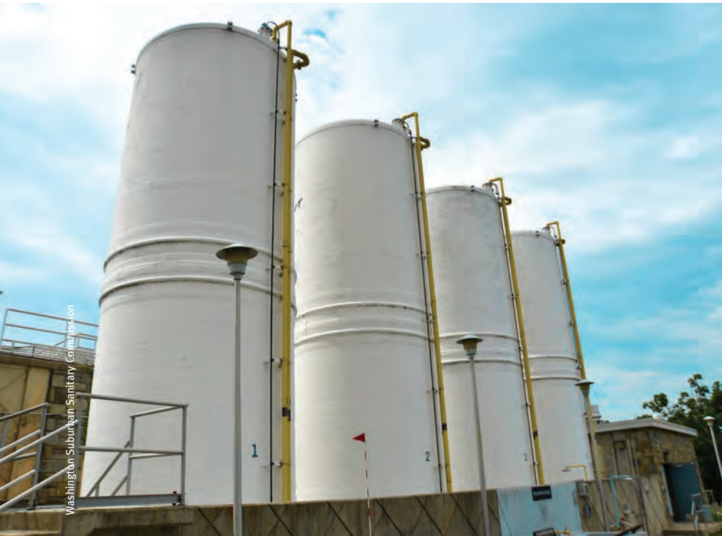
Four 30,000-gallon coagulant (polyaluminum chloride) storage tanks maintained by the Washington Suburban Sanitary Commission
