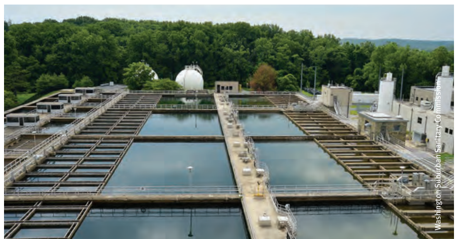
Sedimentation basins and filters at the Washington Suburban Sanitary Commission in Maryland, one of the nation’s largest water utilities.
